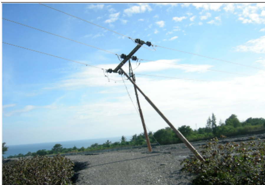
Figure 9 – Transmission poles in Timor Leste after a storm. Source: Baker and Week 2012.
